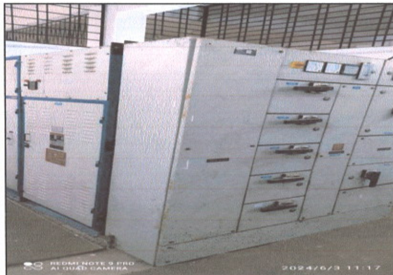
Power room at the basement (105)
