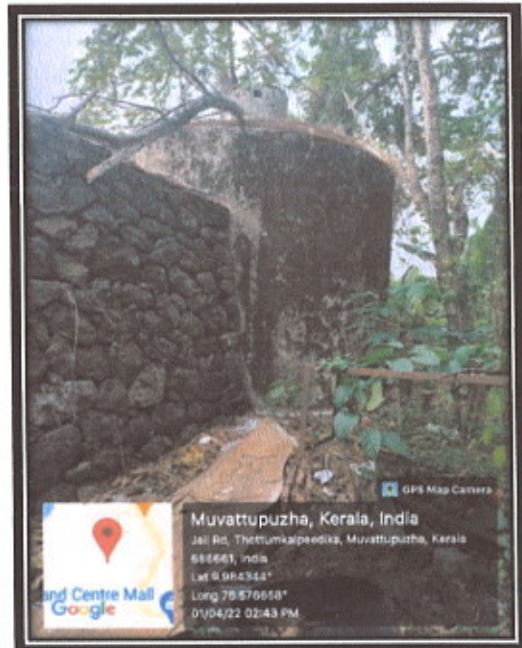
Rain Water Harvesting Storage Tank
